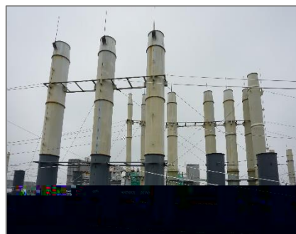
Air Emissions Outlets
